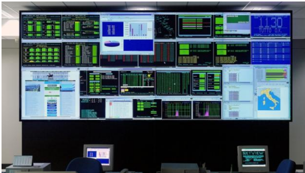
Network Operations Center
